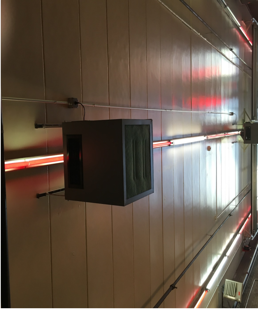
Photo # - 2. This picture is of one of the main electric unit heaters which heat the engine bay area.
