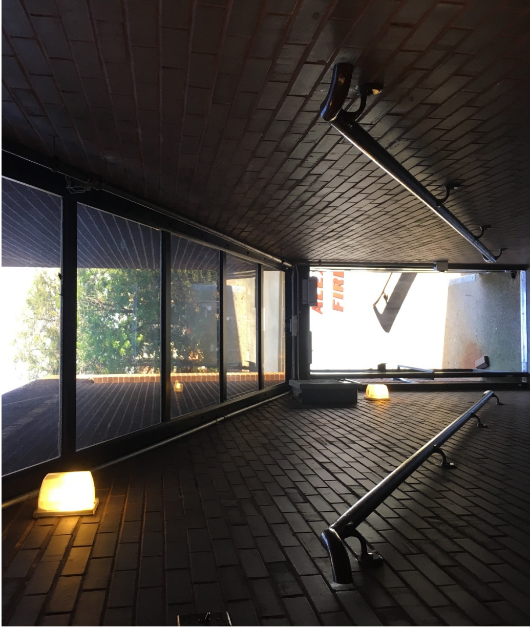
Photo – 13. This picture notes the second skylight in the stairwell which is also leaking.
