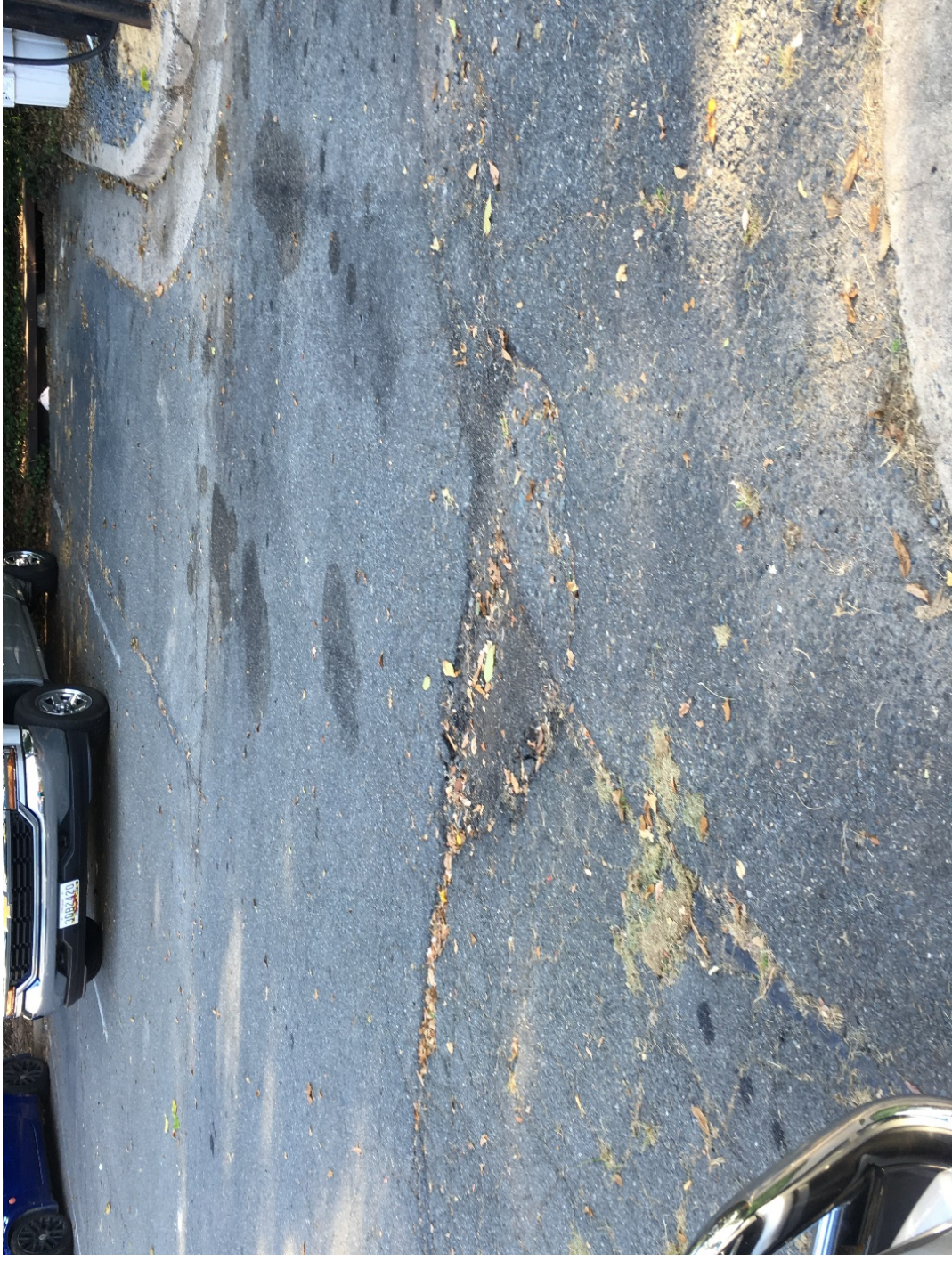
Photo – 15. This picture is an example of the cracked and damaged asphalt at the parking lot area.
