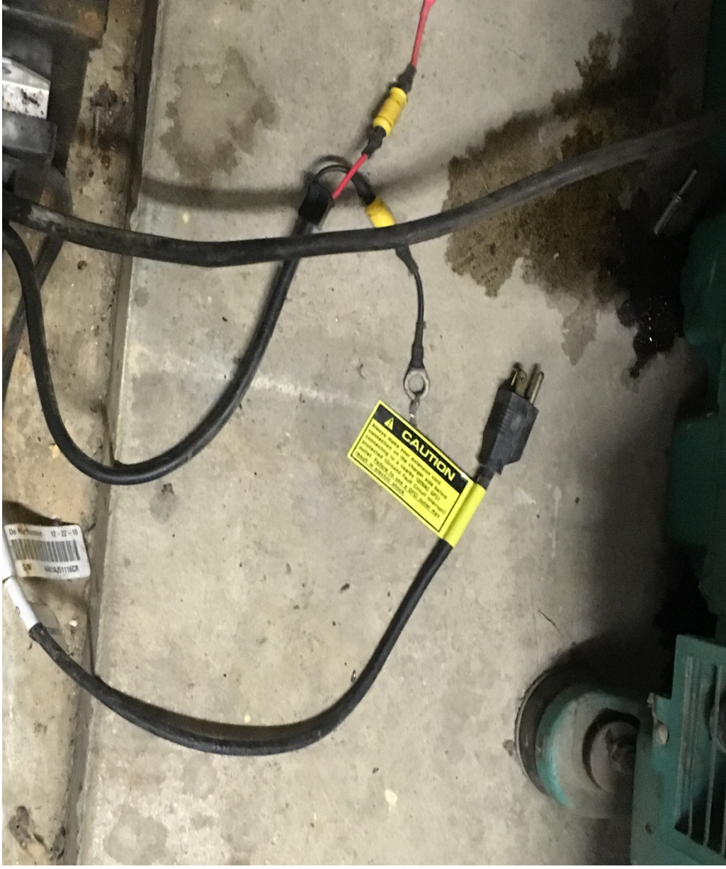
Photo # - 7. This picture is of the power disconnected from the emergency generator battery charger.
