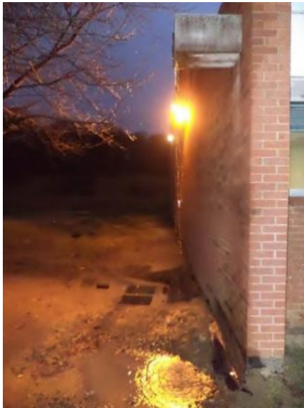
Figure 12: Lack of attachment to foundation drain system.
