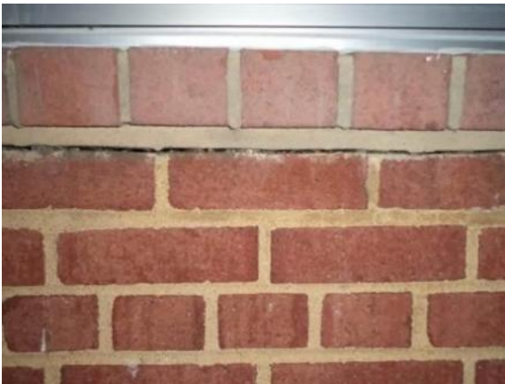
Figure 19: Open mortar joints.
