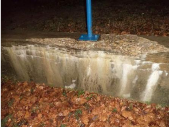
Figure 16: Deteriorated Concrete Retaining Wall.
