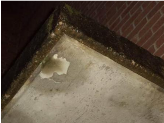
Figure 6: Efflorescence staining at Gym Canopy
