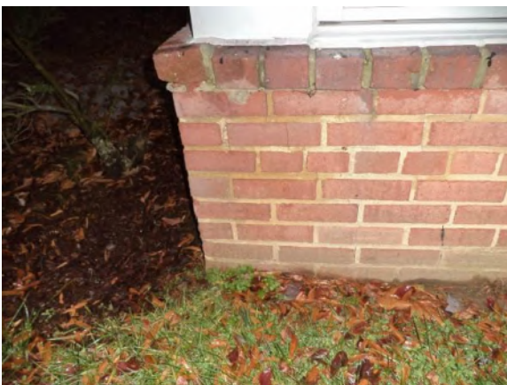
Figure 4: Step Cracking in mortar joint below exposed column (see Figure 5).
