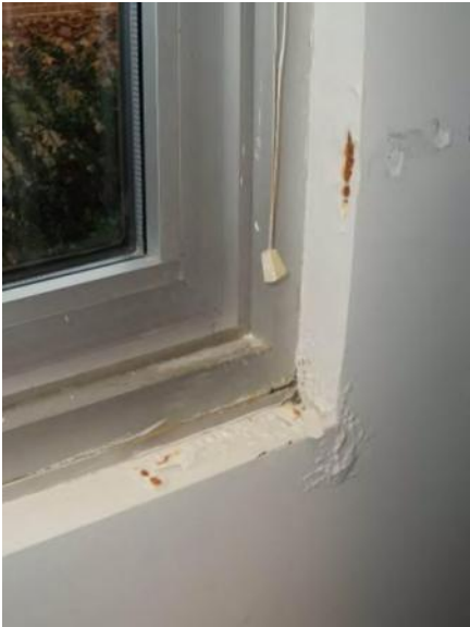
Figure 22: Plaster cracking at window.
