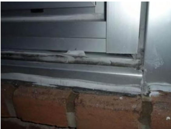
Figure 20: Open joints at windows.
