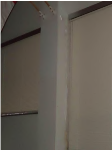
Figure 23: Signs of moisture infiltration at Auditorium Column.
