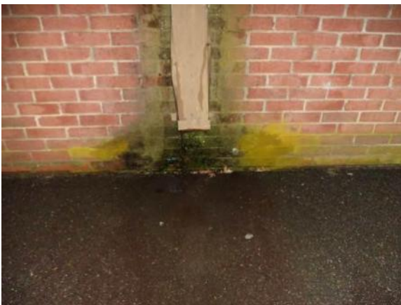
Figure 10: Lack of connection to foundation drainage system.
