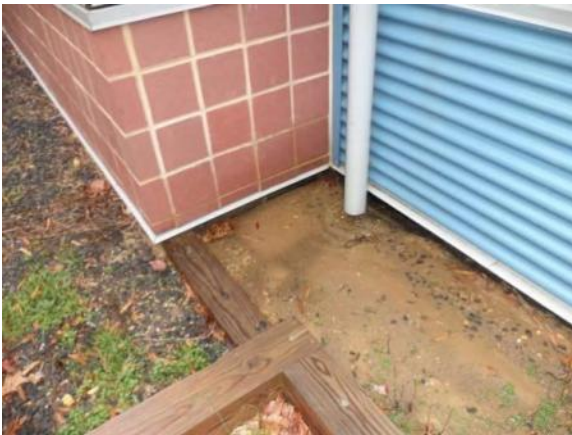
Figure 9: Pooling of drainage at modular foundation walls (clogged)
