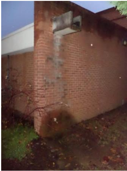
Figure 13: Lack of attachment to foundation drain system.
