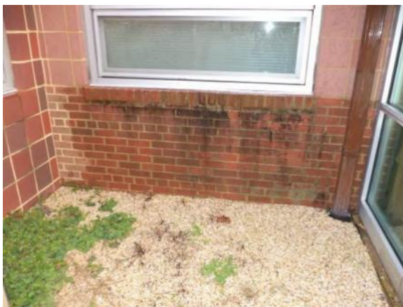
Figure 14: Moisture staining of brick.
