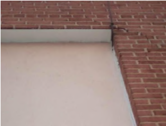
Figure 18: Cracking at lintel steel lintel bearing.
