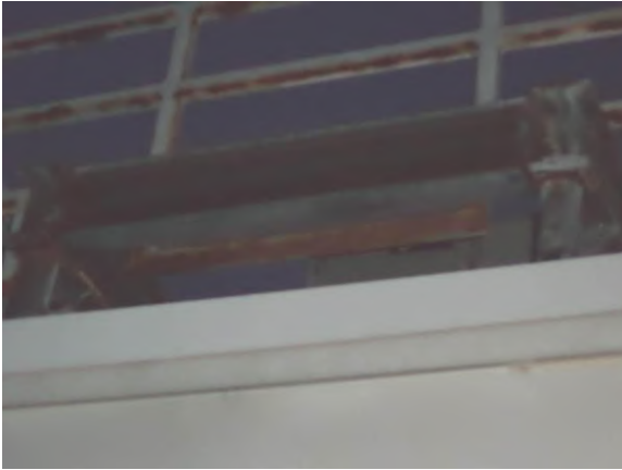
Figure 2: Deterioration of MEP roof top steel.
