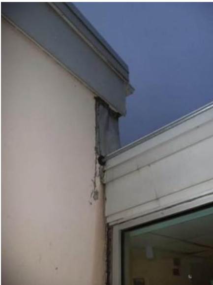
Figure 17: Deteriorated Flashing at Bldg Return.
