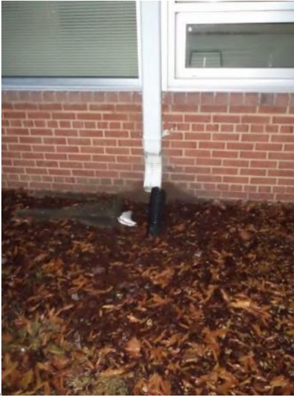
Figure 11: Inadequate attachment to foundation drain.
