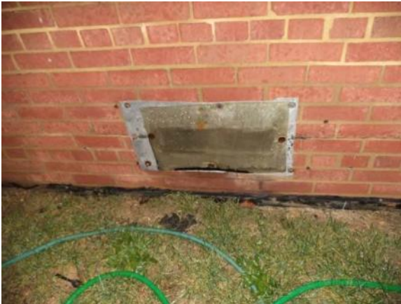
Figure 21: Unventilated crawl space.
