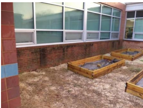
Figure 15: Moisture staining of brick
