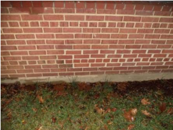
Figure 8: Negative Drainage & Exposed Foundation Wall.
