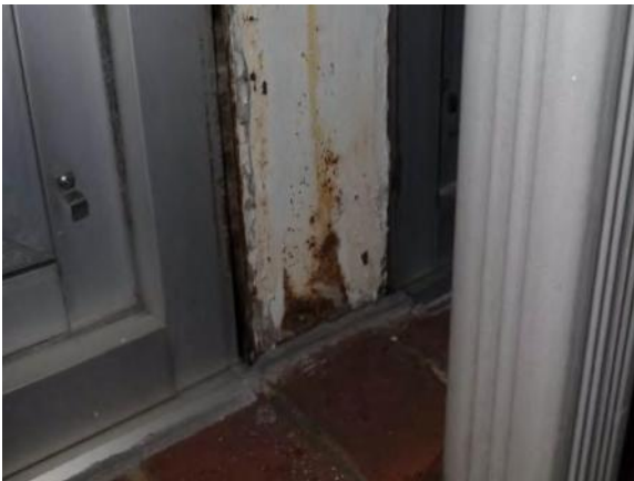
Figure 3: Deterioration of exposed structural steel col.
