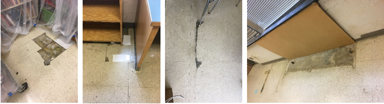
Classroom flooring wear & rear – refer to matrix
