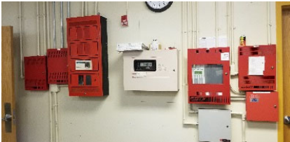
FIRE ALARM CONTROL PANEL
