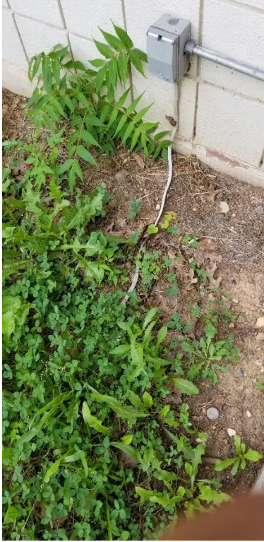
Figure 14: Exposed Wiring to Parking Lot Light Fixture
