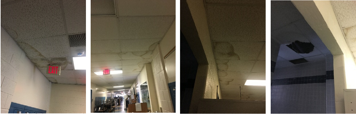
Figure 2. Ceiling stains from roof failure
