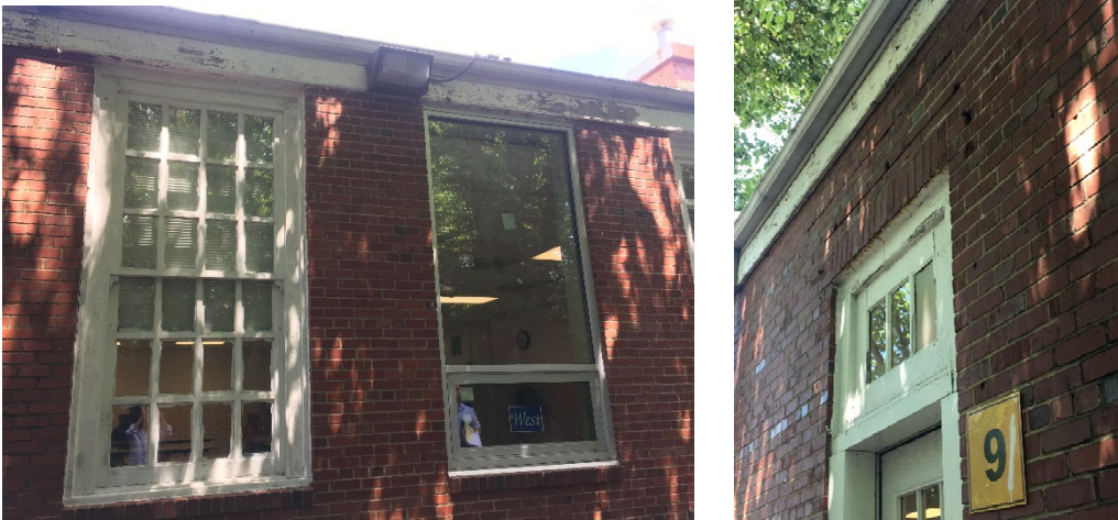
Figure 22 Wood Rot on Windows Due to Moisture
