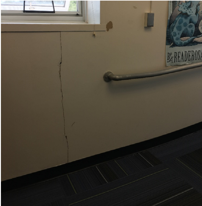
Figure 9 Settlement Crack (seen in Library)
