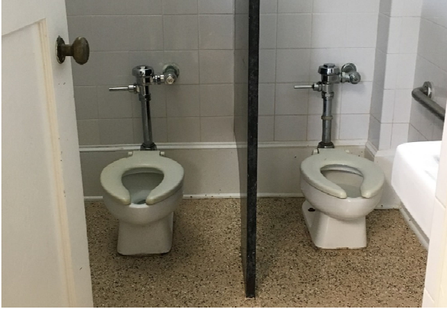
Figure 8 No Stall Doors
