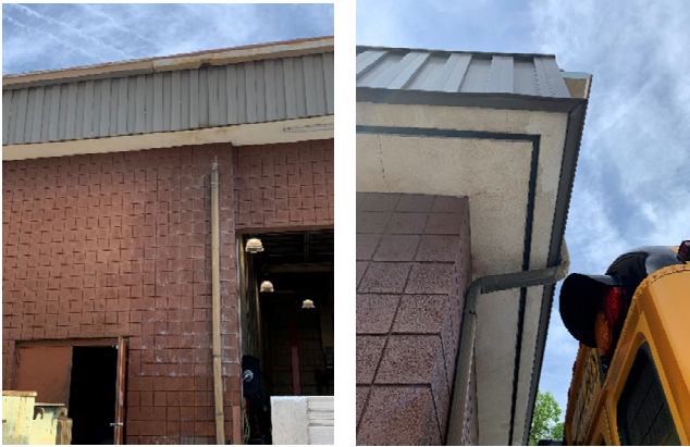
Figure 2. Exterior water damage due to roof drainage failures
