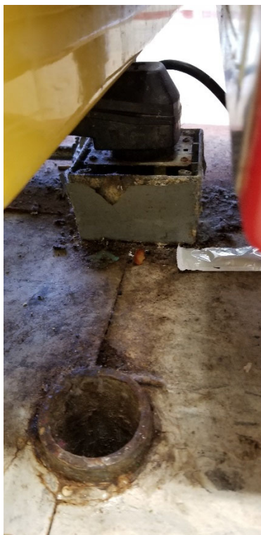
Figure 12: Cafeteria Service Counter – Floor Outlet Missing Cover Plate
