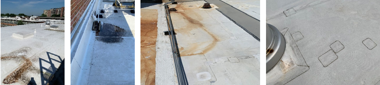
Figure 1. Roof – shown: D wing roof failures and patchwork
