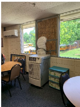
Figure 4: Patchwork measures to correct HVAC inadequacies
