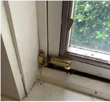
Figure 16 Inoperable Window Hardware
