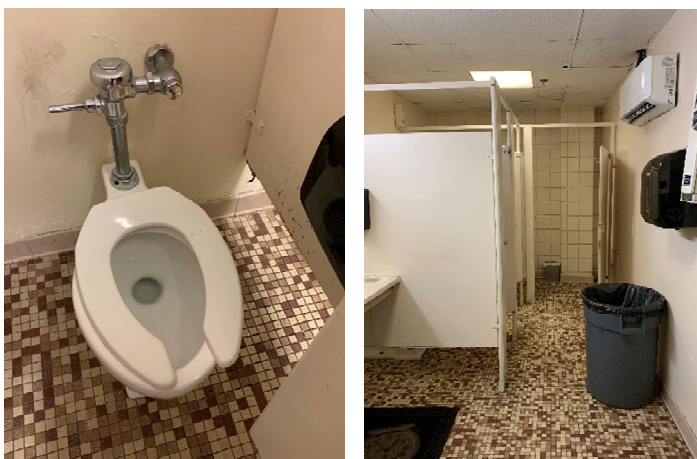
Figure 5: Women's Bathroom – Examples of water damage from leaks
