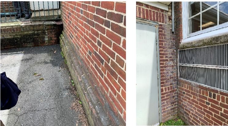
Figure 15 Exterior Wall Moisture and Settlement Cracks
