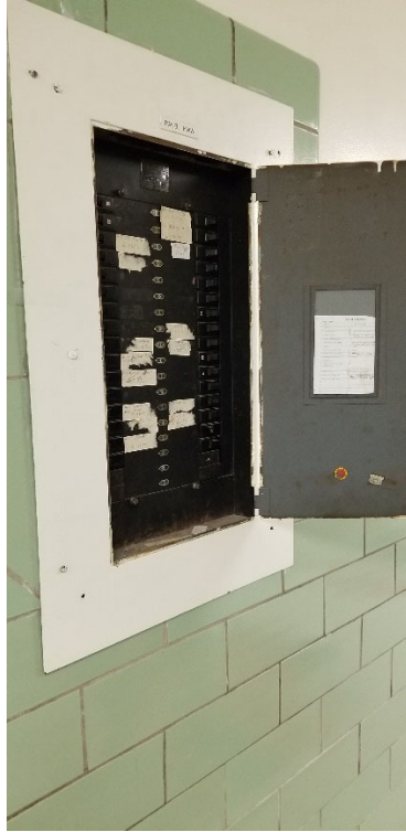
Figure 13: Obsolete Panel 1-WW
