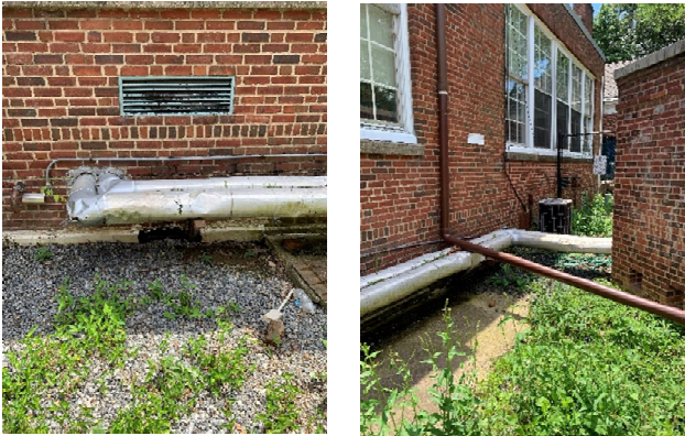
Figure 17 Inadequate Stormwater Drainage
