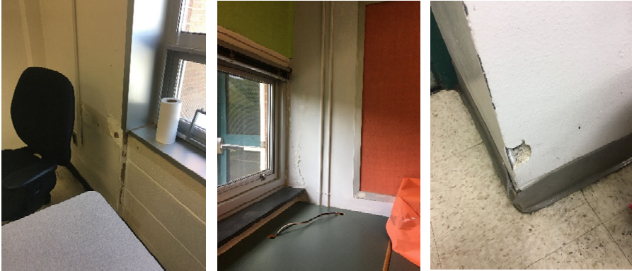
Classroom wall finish issues – refer to matrix
