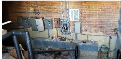
DUST COLLECTOR ROOM
