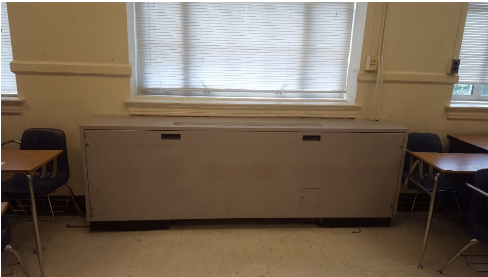
Unit ventilator found in room A310.
