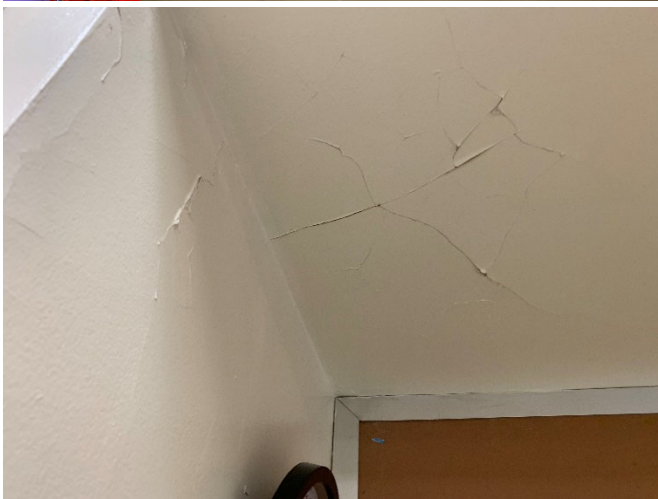
Figure 9: Wall finish issues
