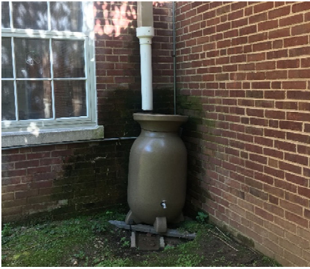
Figure 3 Greywater Collection is Poorly Set
