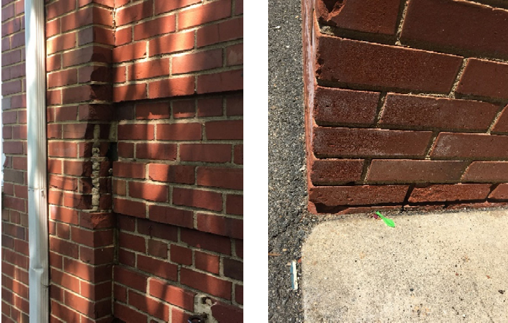
Figure 21 Exterior Walls (weathering and mortar vanishing)
