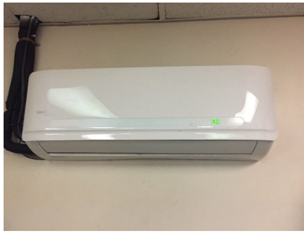
SPLIT SYSTEM AIR CONDITIONER
