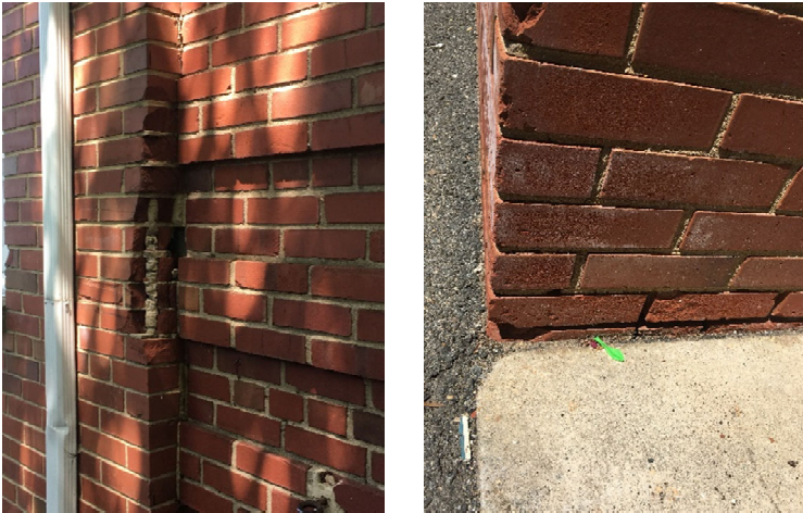
Figure 21 Exterior Walls (weathering and mortar vanishing)
