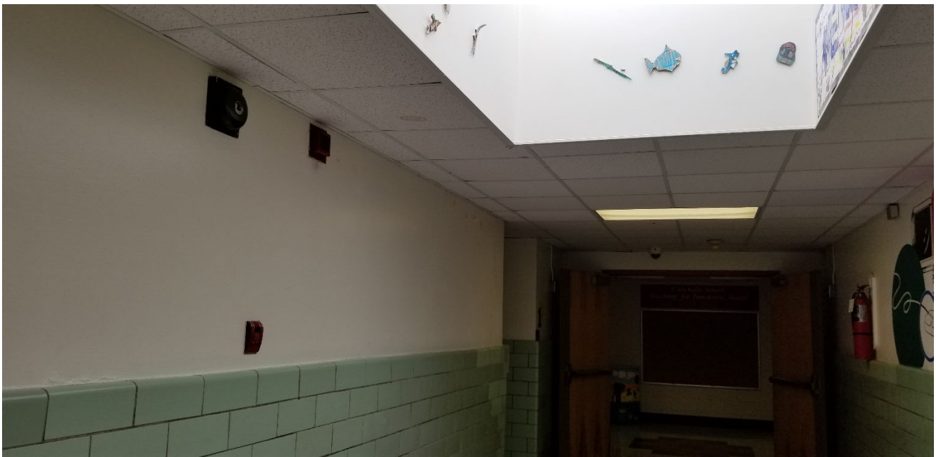
Figure 11: Fire Alarm Pull Station / Horn / Bell – No Strobes or Emergency Battery Pack
