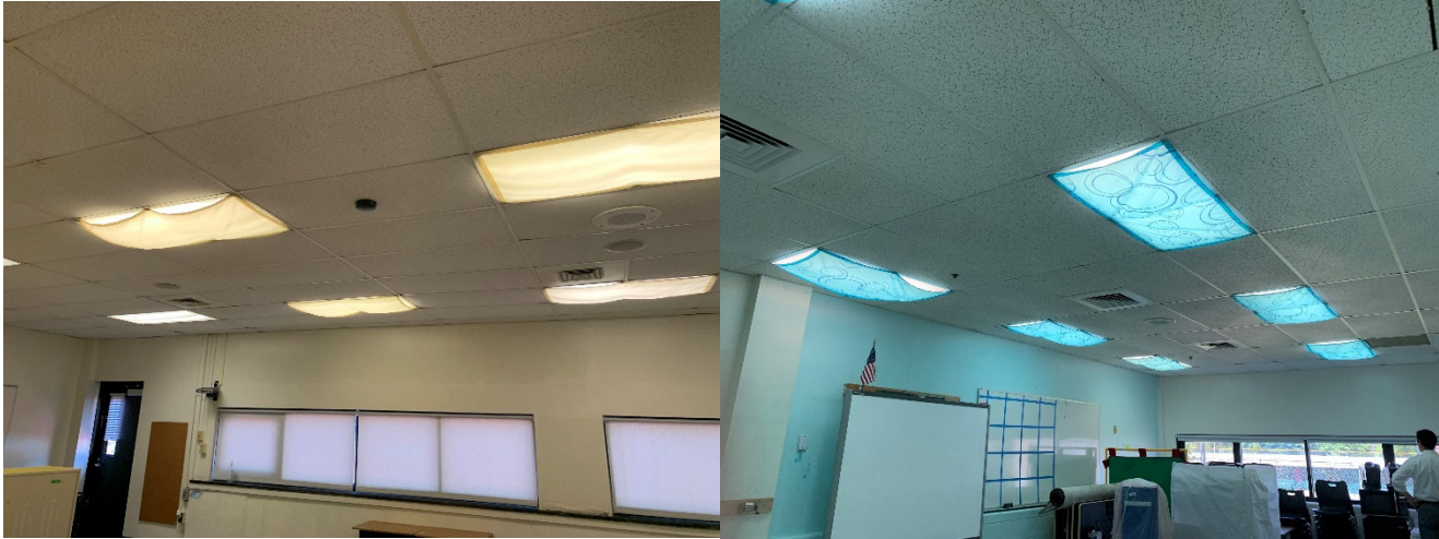
Figure 10: Light dimmers required
