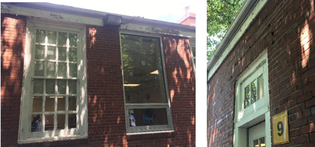
Figure 22 Wood Rot on Windows Due to Moisture
