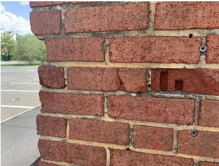
Figure 3: Joint repair needed
