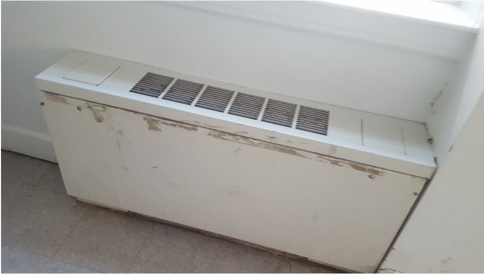
Fan coil unit found in room A113.
