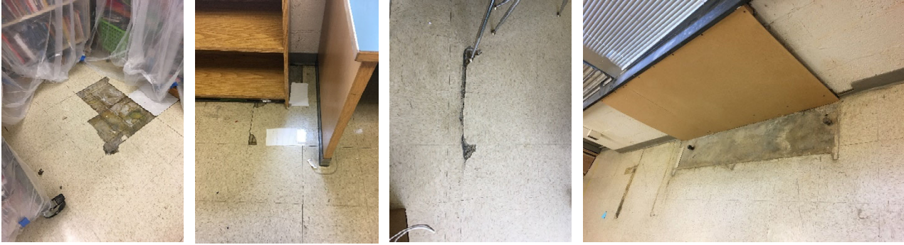
Classroom flooring wear & rear – refer to matrix
