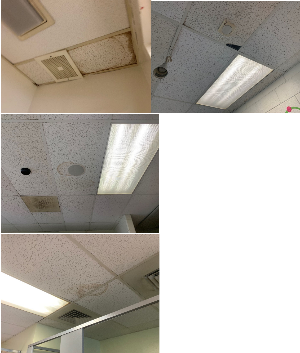
Figure 5: Leaks and staining on ceiling tiles
