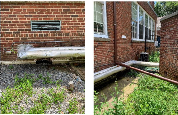
Figure 17 Inadequate Stormwater Drainage
