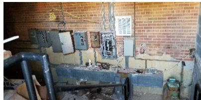
DUST COLLECTOR ROOM
