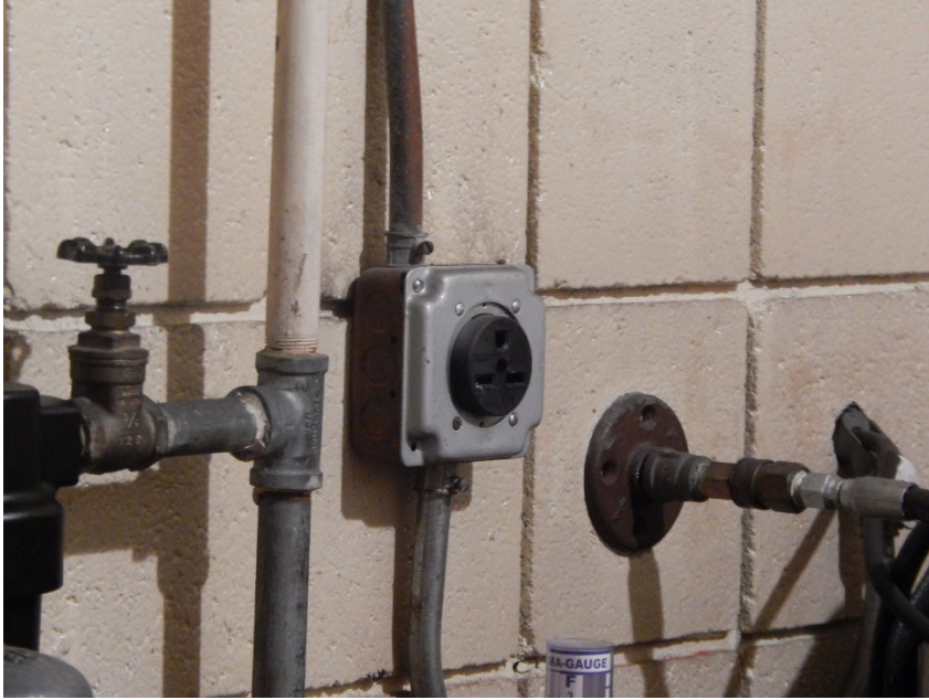
Figure 10: Non-Explosionproof Outlet Located in the Flammable Liquids Storage Space
