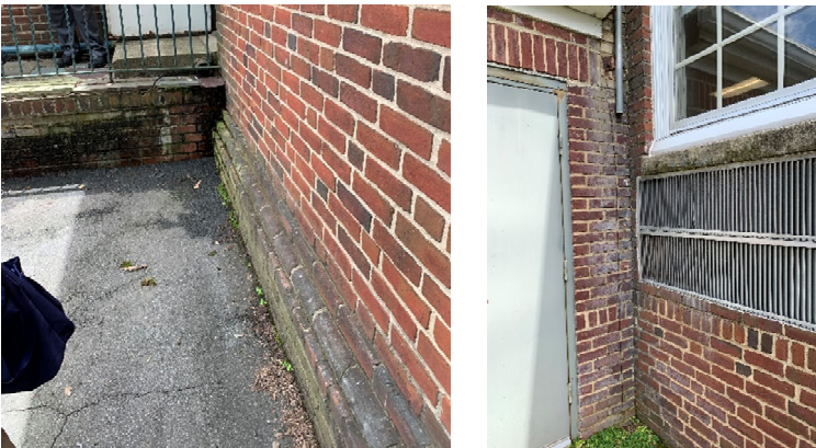
Figure 15 Exterior Wall Moisture and Settlement Cracks
