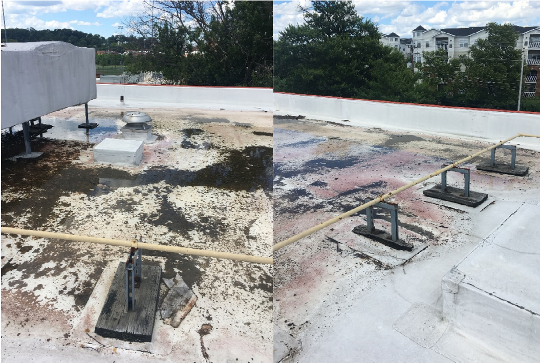
Figure 8 and 2: Water ponding on the roof causing leaks
