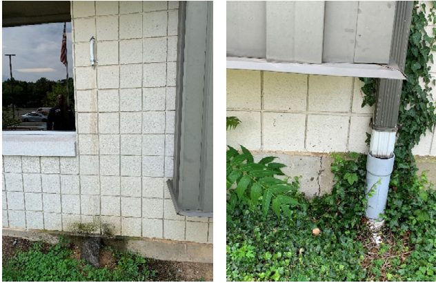
Figure 3: Examples of water infiltration and subsurface breaches in exterior enclosure
