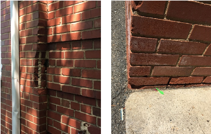
Figure 21 Exterior Walls (weathering and mortar vanishing)
