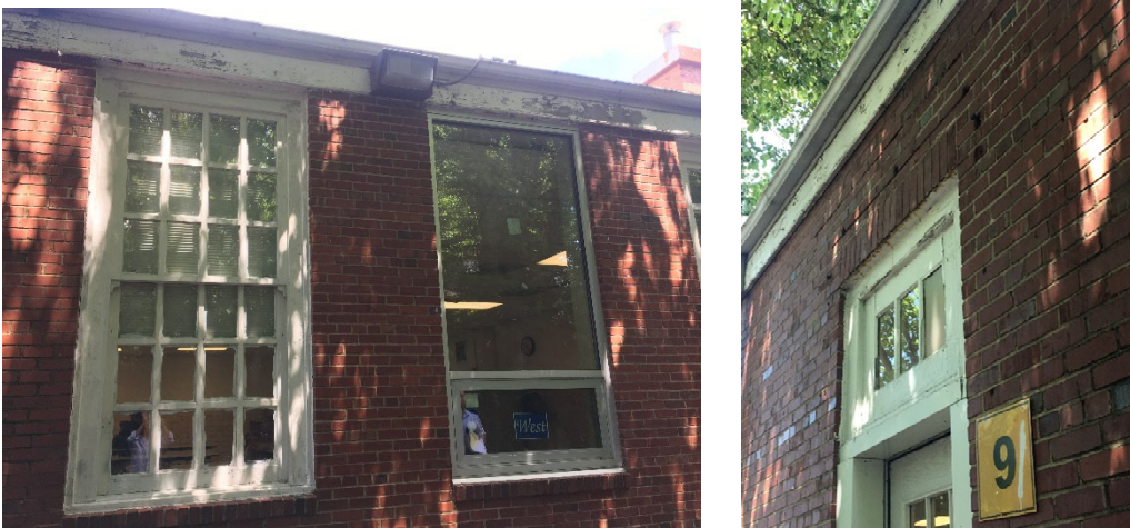
Figure 22 Wood Rot on Windows Due to Moisture
