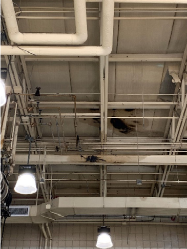
Figure 9: Example of leaks prevalent in high bus bays
