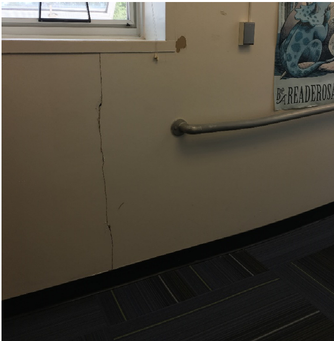
Figure 9 Settlement Crack (seen in Library)
