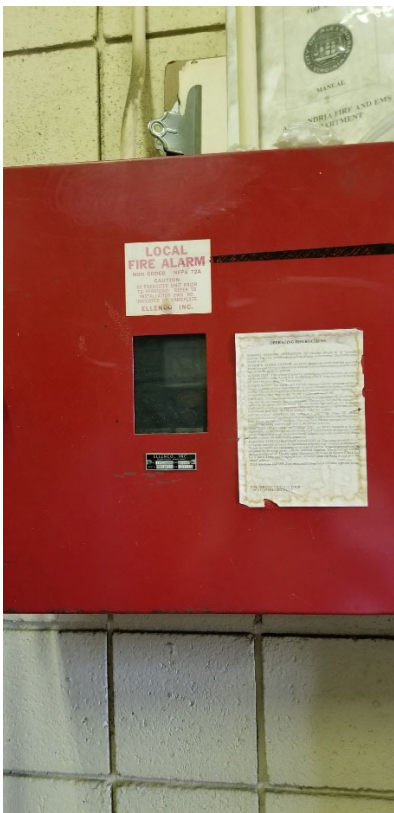
Figure 10: Fire Alarm Control Panel – Local Alarm Only
