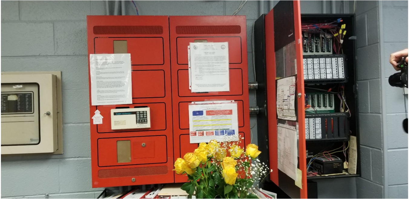
Figure 10: Fire Alarm Control Panels
