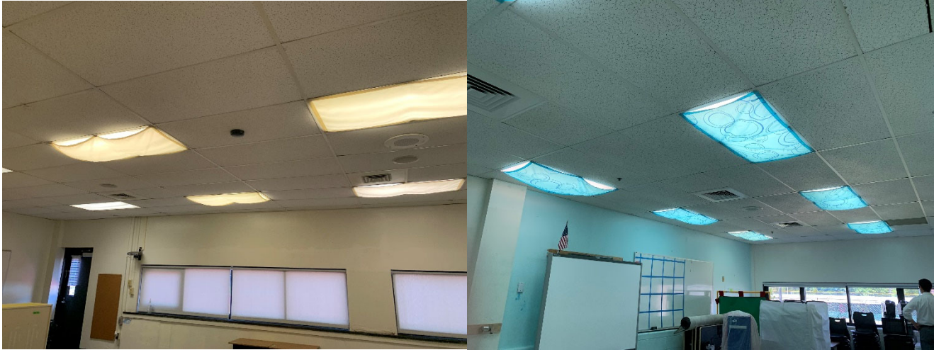
Figure 10: Light dimmers required
