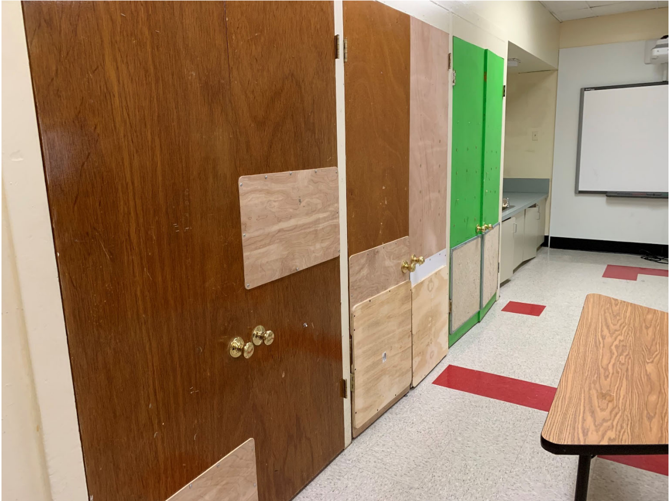
Figure 9: Furniture laminates damaged
