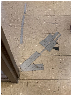
Figure 7: Entry area - Damaged floor tiles
