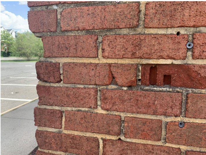
Figure 3: Joint repair needed
