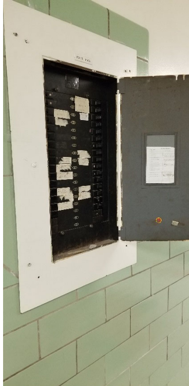
Figure 13: Obsolete Panel 1-WW
