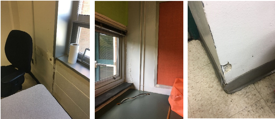
Classroom wall finish issues – refer to matrix
