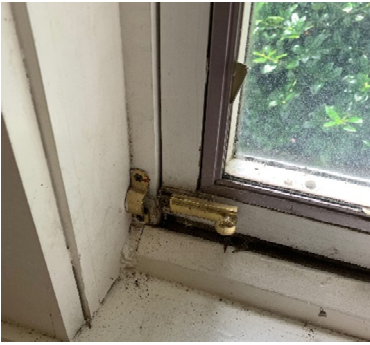
Figure 16 Inoperable Window Hardware
