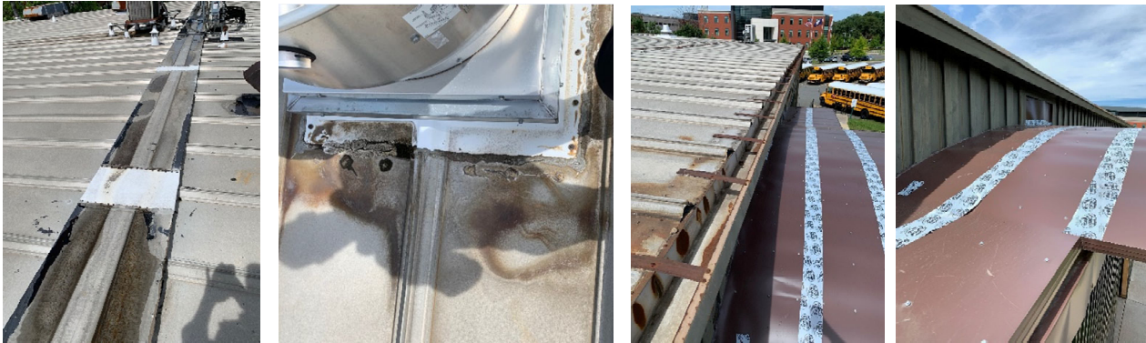
Figure 1. Roof – Leaks, corroded seams and surfaces, gutter detail and incomplete canopy
