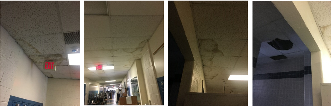
Figure 2. Ceiling stains from roof failure
