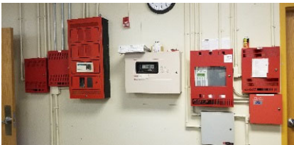
FIRE ALARM CONTROL PANEL
