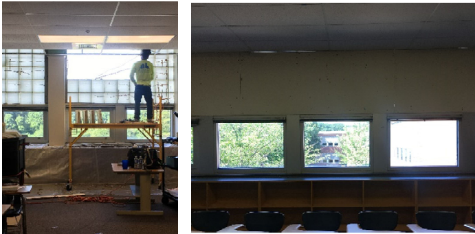
Figure 8. Window replacement (Left to right) E wing in progress and B wing soon to commence .
