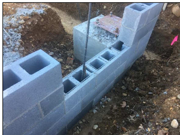
CMU wall being installed upon building footer and around corner support concrete footer.
