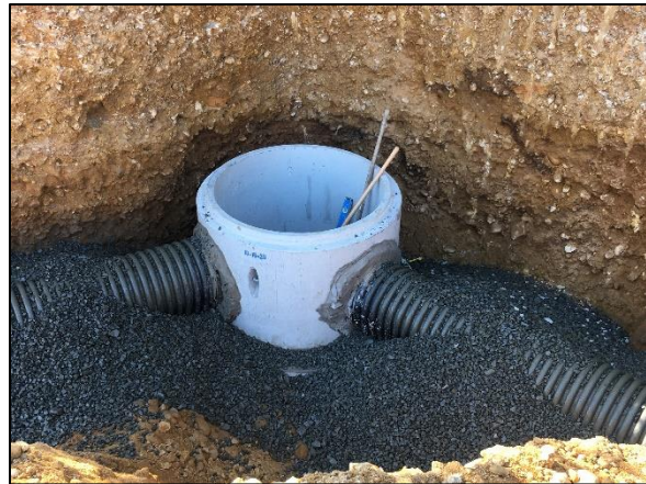
Sanitary flex PVC piping and concrete sewer doghouse structure.
