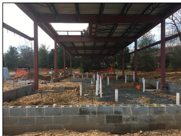
Steel supports and steel roof deck over foundation walls and plumbing stub-outs.
