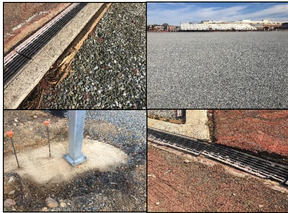
Clockwise top left: rotted header board, gravel base, field drain, awning footer/support.
