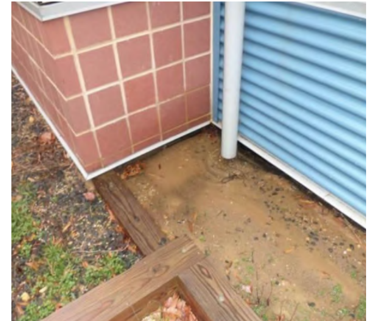
PONDING WATER AT FOUNDATION
