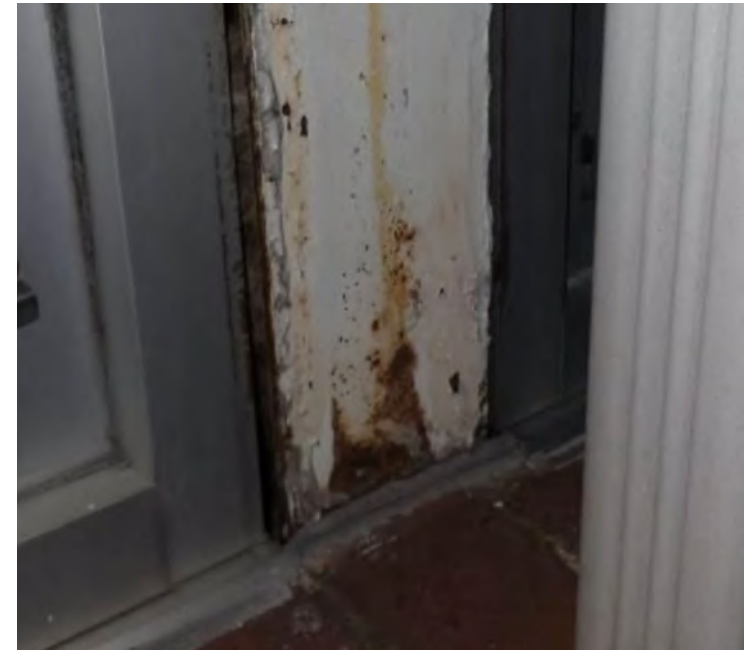
DETERIORATION OF EXPOSED COLUMN
