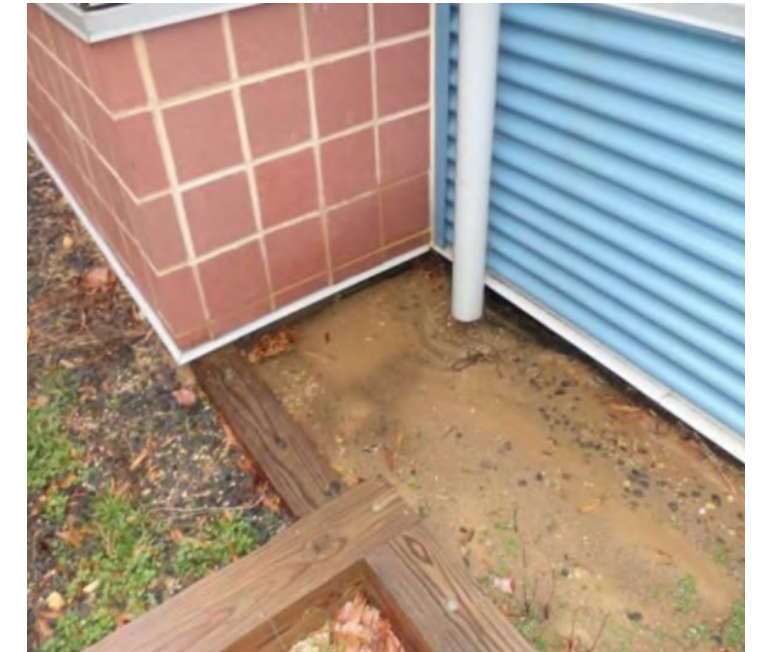
PONDING WATER AT FOUNDATION
