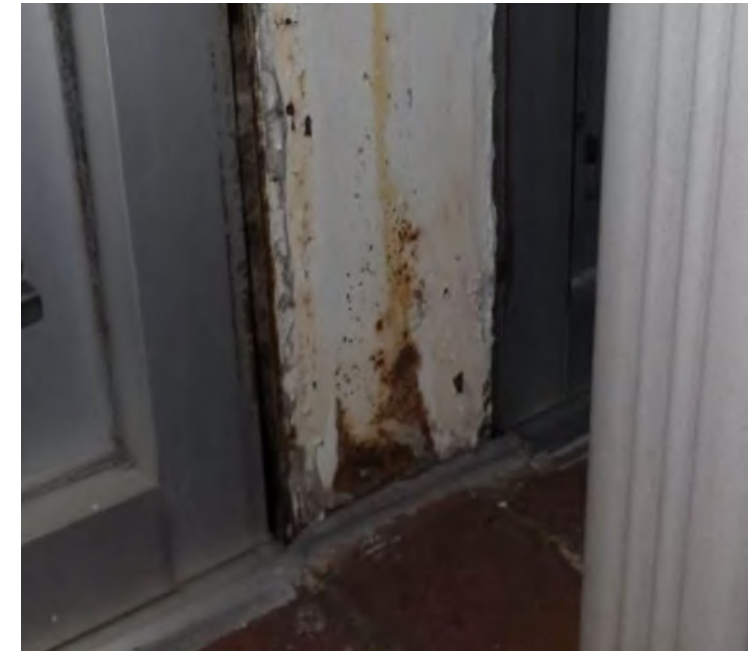
DETERIORATION OF EXPOSED COLUMN
