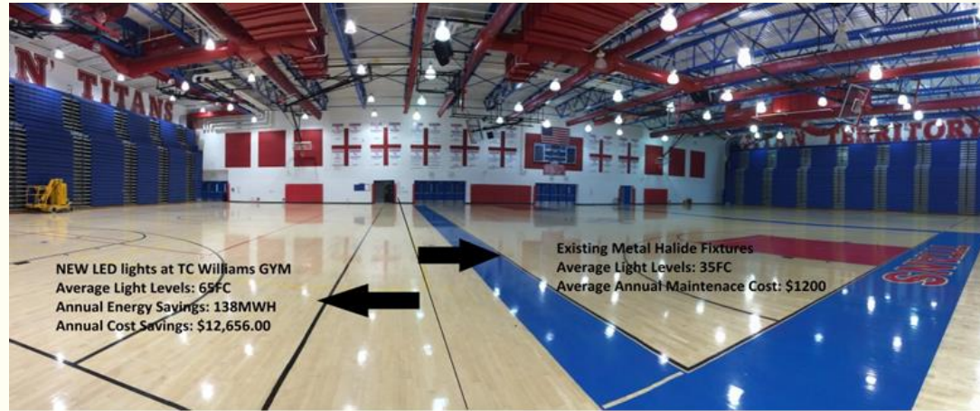
T.C. William Gymnasium – Annual energy savings - 138 MWH, Annual Cost Savings - $12,656
